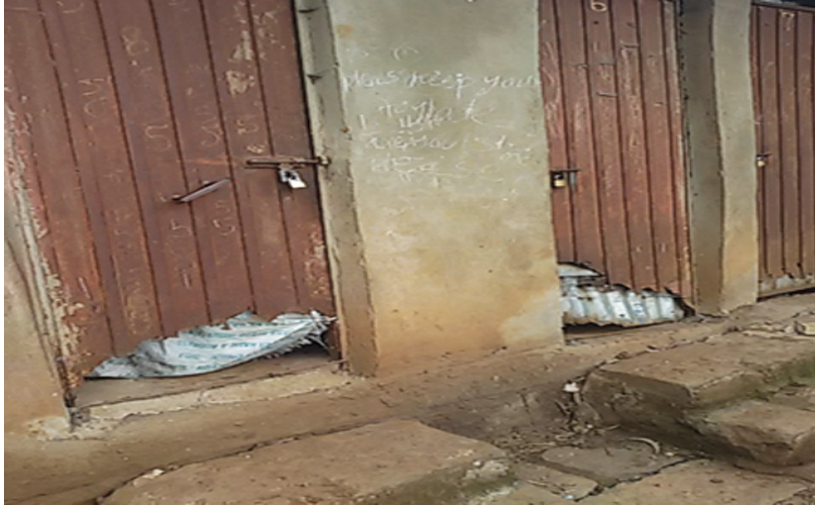
Figure 19: Shared latrines, sandwiched in between houses in collapsing superstructures, are overused and overflowing with raw sewage around
