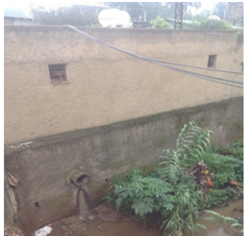
Figure 18: Direct discharge of waste water from Abebech Gobena Hospital to Kurtume river
