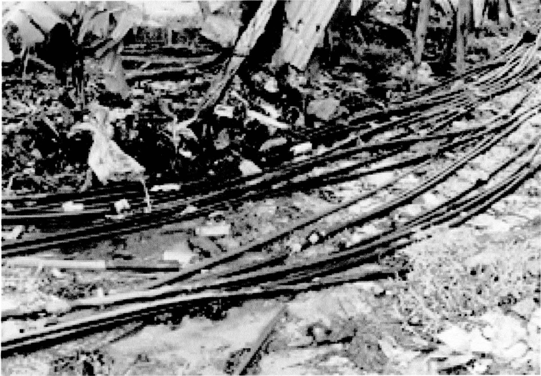
Figure 2: Plate “A” – Presents typical picture of leaking pipes at the project site
